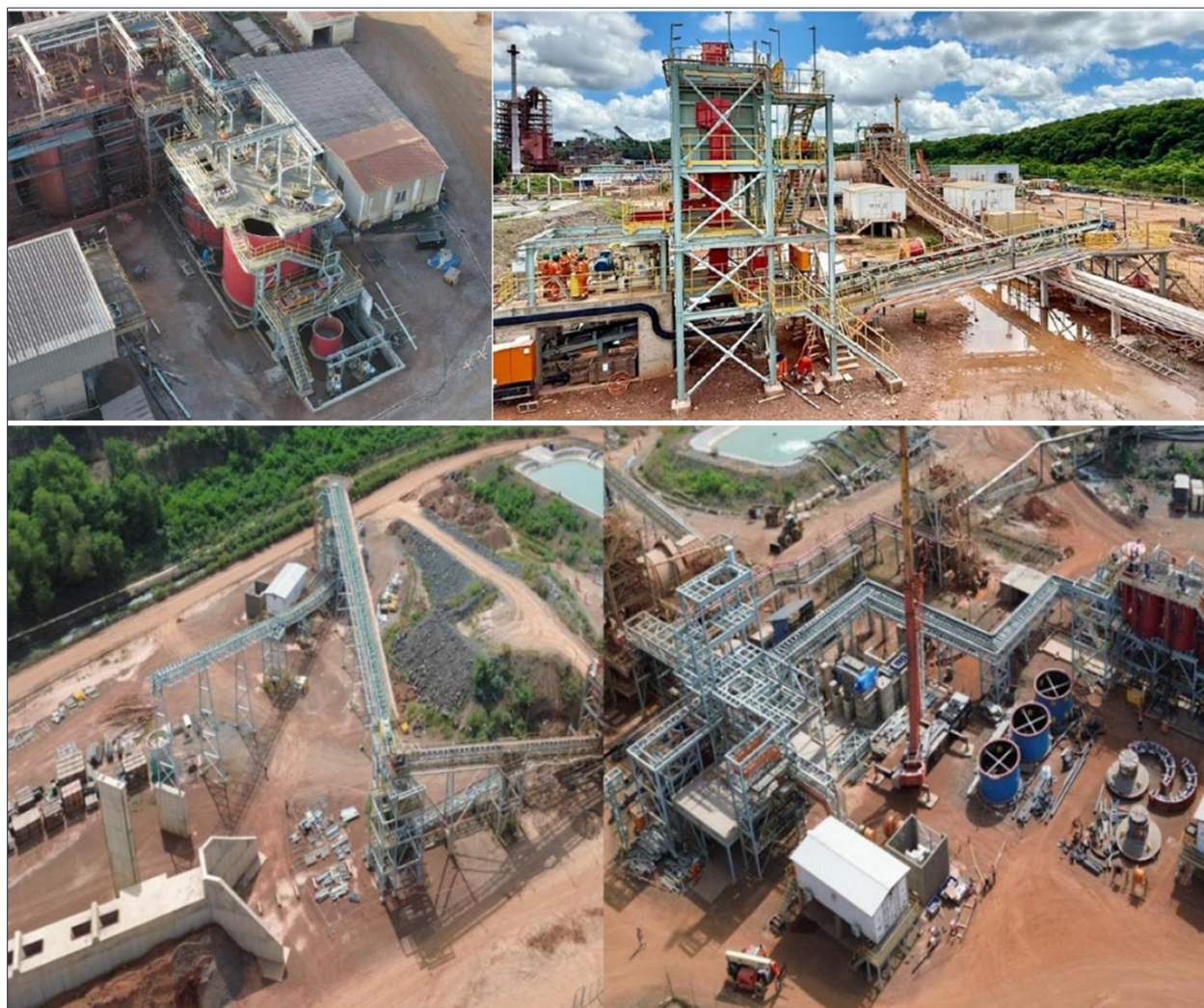
Figure 3. SSPC (A) CCIL circuit, (B) Pebble Crusher, (C) Secondary Crushing and (D) Ball Mill areas
