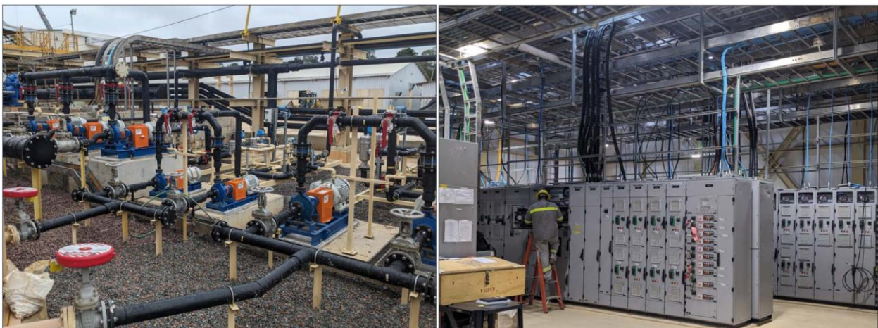
Figure 3. (A) Water services and (B) CIL electrical room
